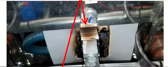
SCR circuit overheated in Torus MPS Insulation burned
